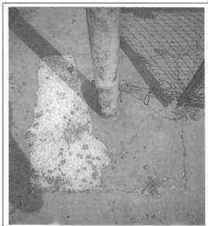
D. Extensive cracking and peeling around square footing for net post.
