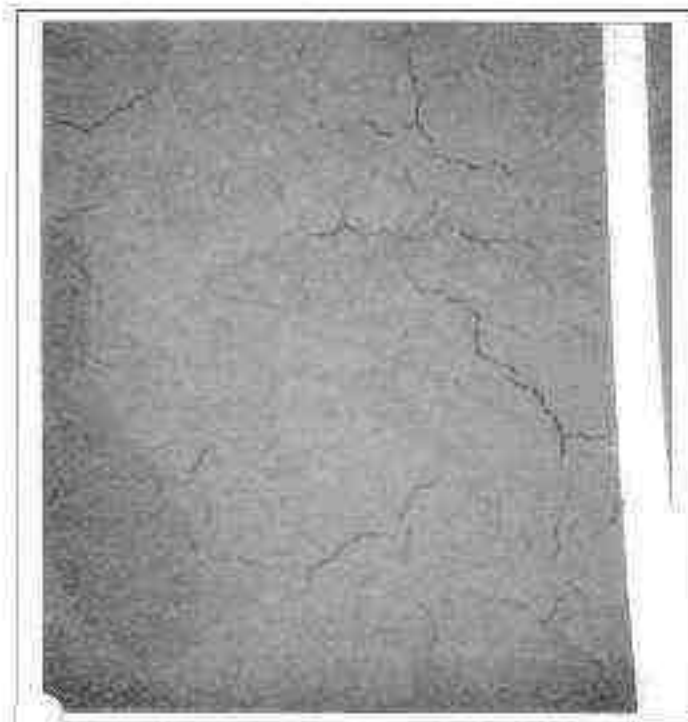
C. Surface cracks - not related to the expansion joints.
